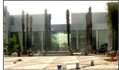
(Pic 4.1) North Lobby Entrance. A car will eventually be displayed on the outside platform shown.
