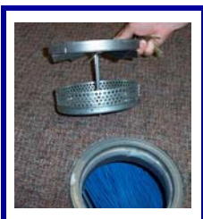
Floor diffuser and cable tray access.
