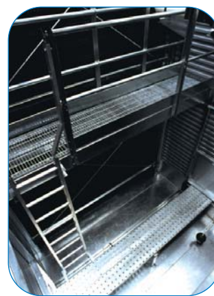
Internal ladder and service platform
