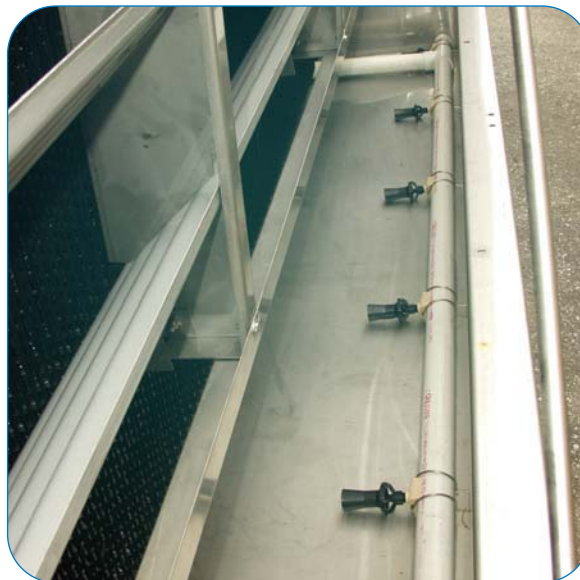
Basin Sweeper Piping
