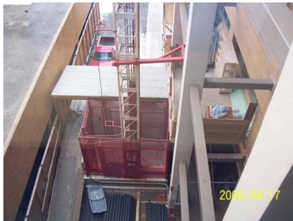
Figure 2 - Material Hoist/Loading Dock
