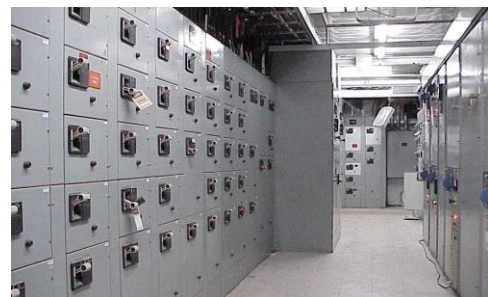
Figure 6: Large-scale motor control center
