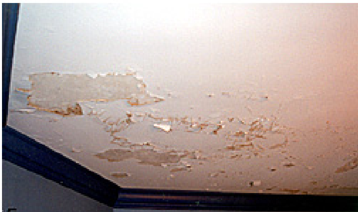
Example of moisture damage to gypsum.
