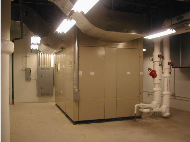
Figure 2.3A. McQuay Packaged SWP Air Handling Unit in Third Floor South Mechanical Room.
