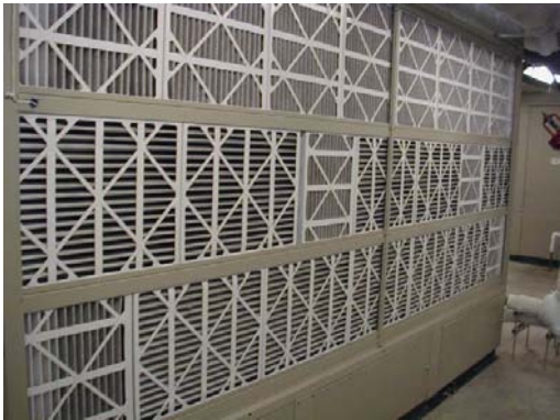
Figure 1.3D. AHU Air Filter.
