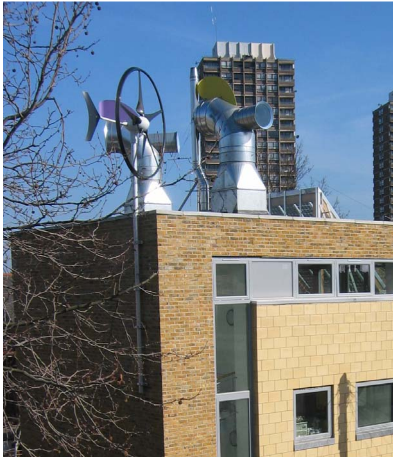
Figure 1 - Installed SWIFT Rooftop Wind Energy System™
