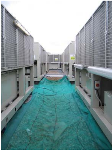
Fig 3.6 Existing Air-Cooled Screw Chillers
