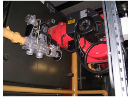
Fig 3.7 Boiler Pump in Rooftop Plant
