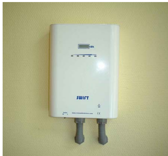
Figure 7 - Installed SWIFT™ Electronic Control System
