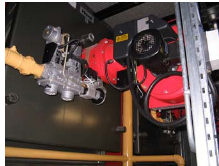
Fig 3.7 Boiler Pump in Rooftop Plant
