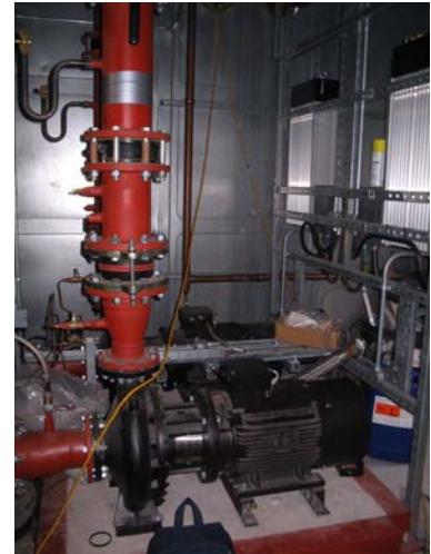
Fig 3.8 Central Boiler Plant
