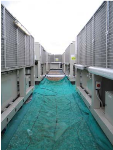
Fig 3.6 Existing Air-Cooled Screw Chillers
