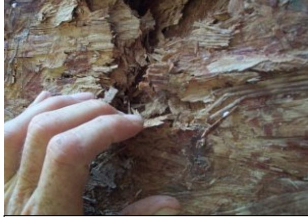
Image 4: Rotten sheathing below the insulation
