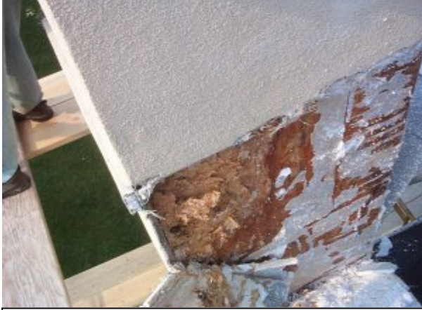
Image 3: Rotten sheathing below the insulation
