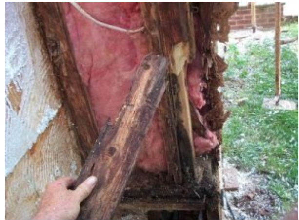
Image 2: Rotten corner post
