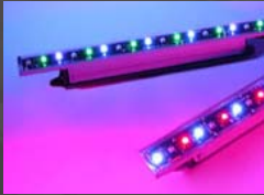
Custom RGB LED fixture recessed in elevator threshold
