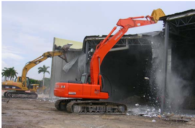
F4. Roof System Removal after Columns & Joists Were Burned
