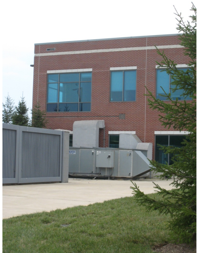
Figure 2 Current Swimming Pool Dehumidifier
