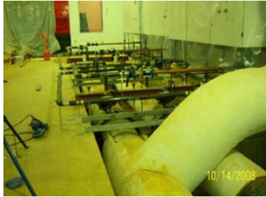
Figure 2 - Mechanical trench in a computer room.
