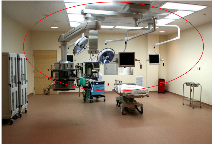
Figure 9: Example of a Typical Operating Room Boom
