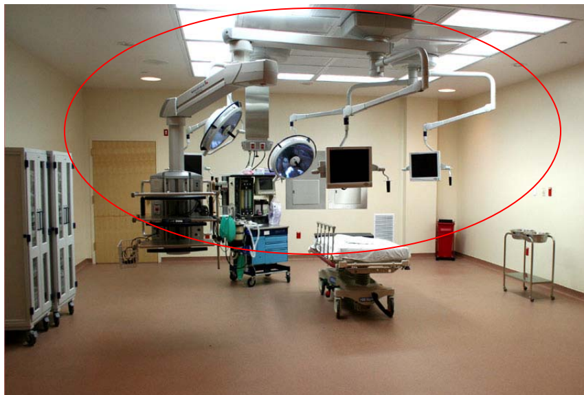
Figure 1: Example of a Typical Operating Room Boom
