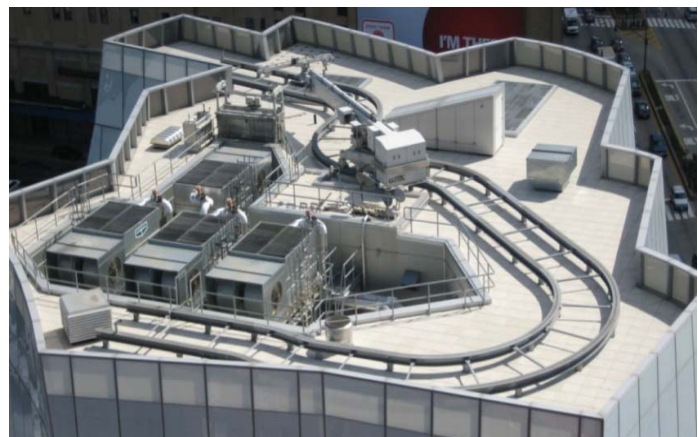
Figure 6: Photo of roof-top, showing mechanical and window-washing equipment
