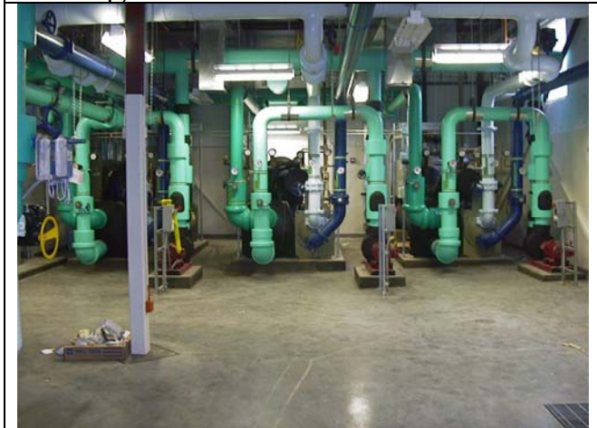
Figure 1-4: Chillers (Courtesy of Tatro Plumbing)
