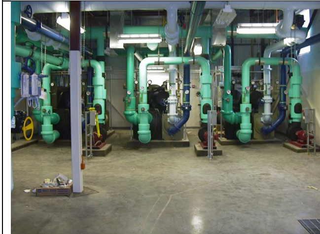
Figure 7-1.2 - Chillers (Courtesy of Tatro Plumbing)
