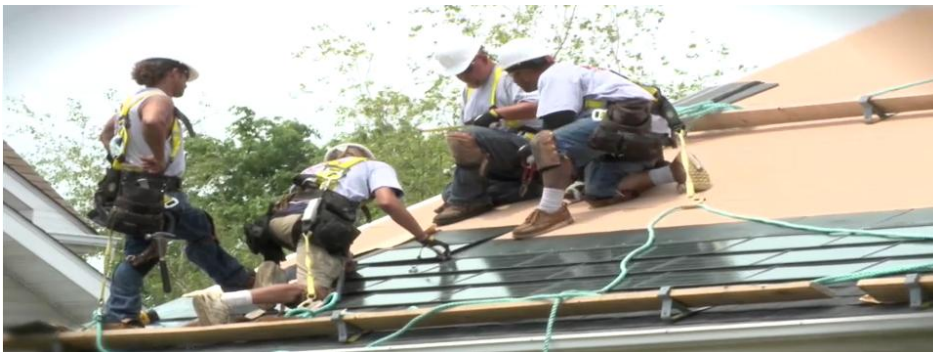
Figure 15: Solar Shingle installation using traditional asphalt shingle pattern (image property of DOW Chemical Company)
