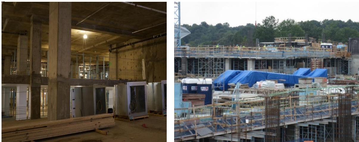
Figure 23: Escalators and Fans Stored on Slabs
