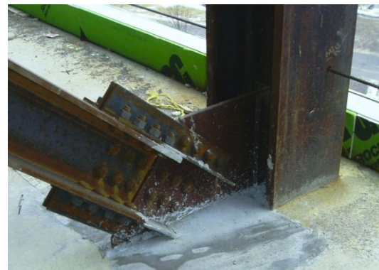
Figure 10 - Diagonal Brace Connection at Column Photo Courtesy of Jim Boje, PE (Wendel)
