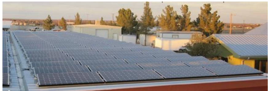
Figure 70.2, Image of installed HIT 220A solar panels. This is how TCMC roof, where solar panels were placed, will look. Image from Panasonic Sanyo HIT Technology
