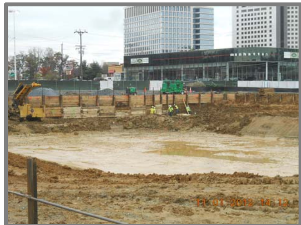
Figure 6.1: Aftermath of Hurricane Sandy on Block 12's building footprint
