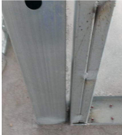
Figure 11: Panels tilted by Uneven Concrete, Down.
