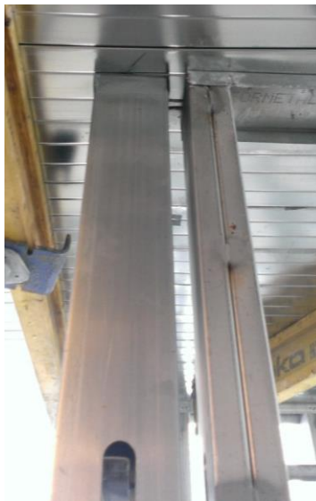
Figure 10: Panels tilted by Uneven Concrete, Up.
