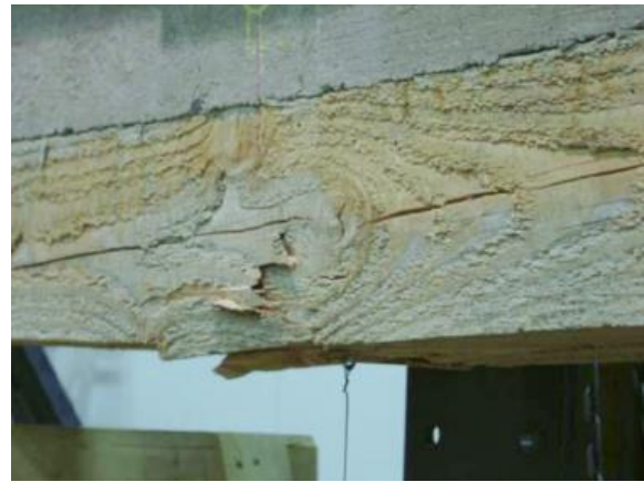
Figure 118: Midspan flexural failure (Balogh et al.)
