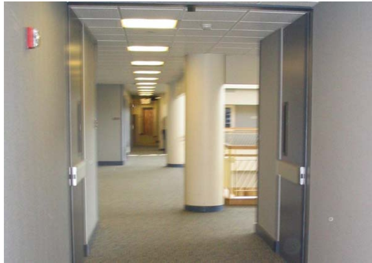
Figure I-3 Concrete columns that serve as the gravity system for The Medical Office Building and an architectural continuation from the existing office buildings
