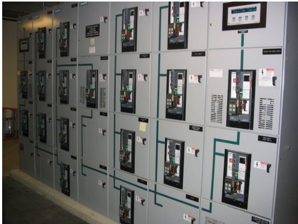
Figure I-6 Switching board for the Medical Office Building
