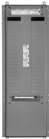
250 A Maximum Main Lugs Trim Installed
