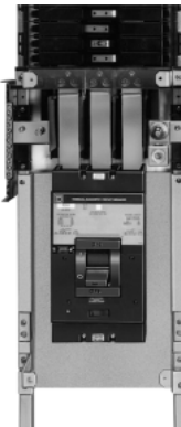
400 A LAL Main Circuit Breaker
