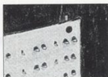
Installation begins with a water infiltration barrier stapled over the substrate. Metal panel is then fastened to the wall.
