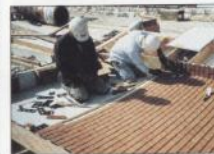
Assembly of brick templates are done on site for Tilt-Up or in a controlled environment.
