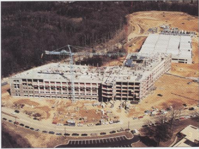
Multiple angles and curved walls were designed for this U.S. Naval Air Systems Command Facility to resemble a Stealth aircraft when viewed from overhead.
