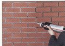
Mortar is installed into the brick joints with a grout bag or with mortar dispensing gun.
