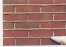
After adequate time has been allowed for mortar to set, mortar is applied with a grout bag.
