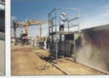
After installation, templates are removed and walls are cleaned with high pressure water.
