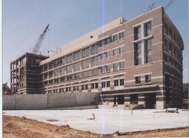
Large panels were constructed off site in a controlled environment. Using cranes to hang the panels allows for quick and efficient installation.
