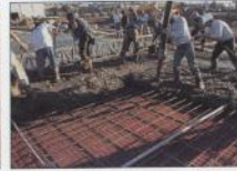
Concrete is poured and vibrated to insure mortar joints are filled properly.
