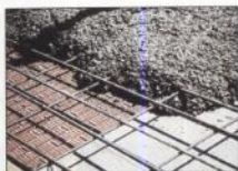
After steel reinforcing is in place, concrete is poured over the assembly.
