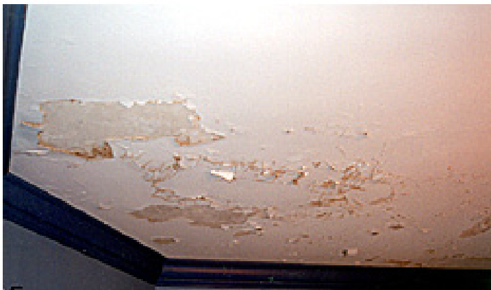
Example of moisture damage to gypsum.
