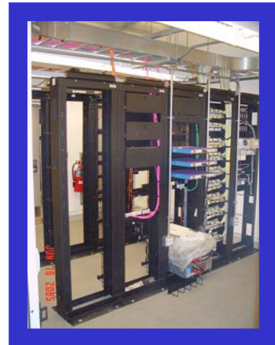
Figure 3 – A telecommunication closet from Wedge 2, which looks similar to the design for Wedge 3.
