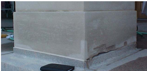
Figure 4 - An example of poorly matched limestone patching on an historic mall entrance column.
