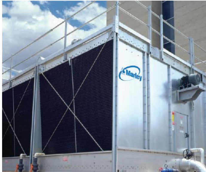
Figure 2 - Marley Cooling Tower
