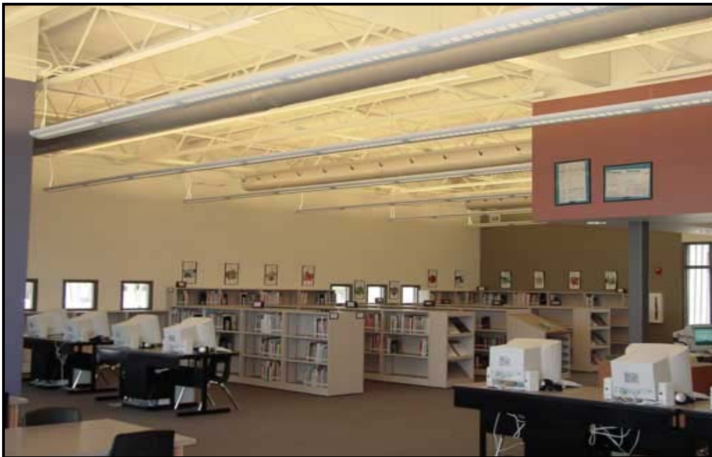
DuctSox in Franklin County Library
