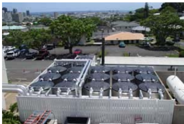
Figure 13: Calmac IceBank Storage Tanks
