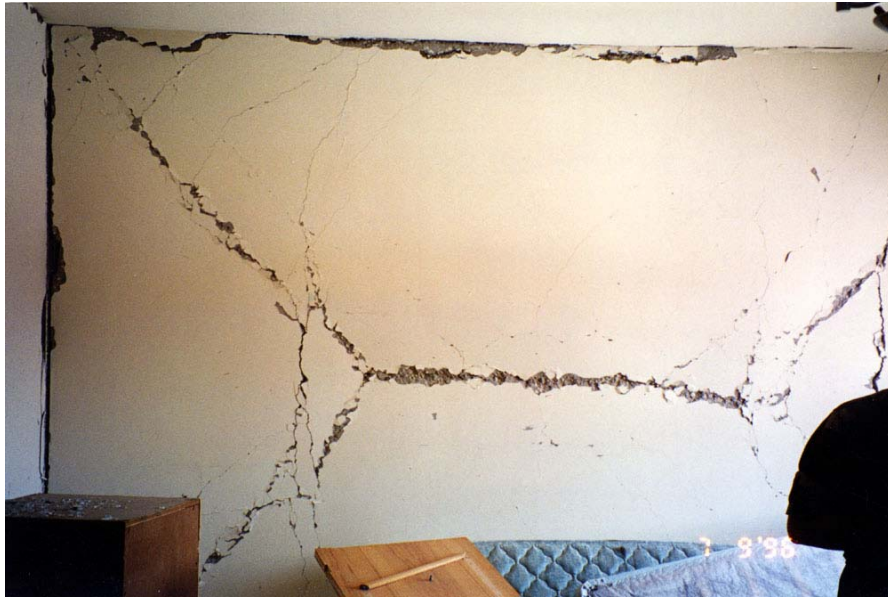
Figure C22. Interior wall exhibiting yield line damage
