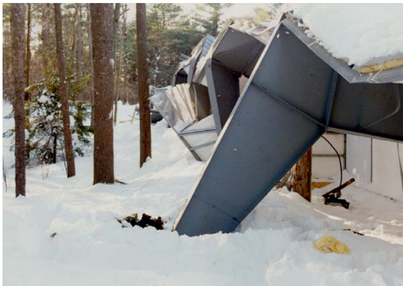
Figure C10. Failed bents looking in direction of progression of collapse
