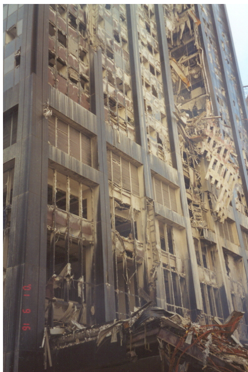
Figure C16. Gash in North Face of 130 Liberty Street
