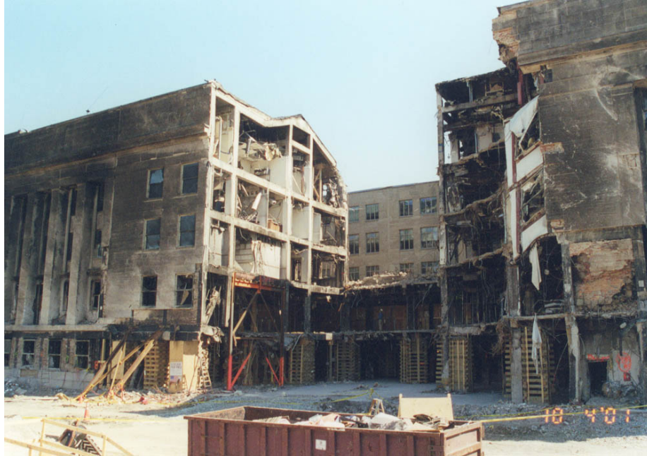
Figure C14. Collapse area after debris removal
