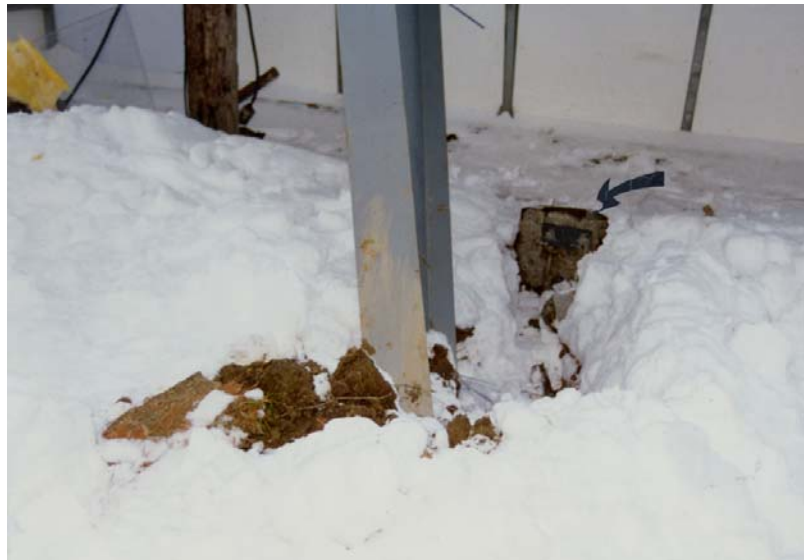
Figure C11. Split pier (arrow) at failure initiation location
