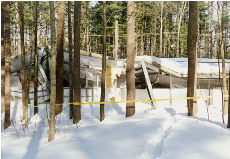
Figure C8. Collapsed Jackson Landing Skating Rink
