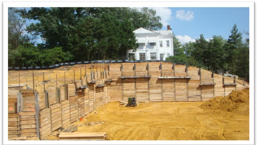
Figure 6: North Hall Soldier Beams, Lagging and Tiebacks Photo Taken By: Brandon Tezak
