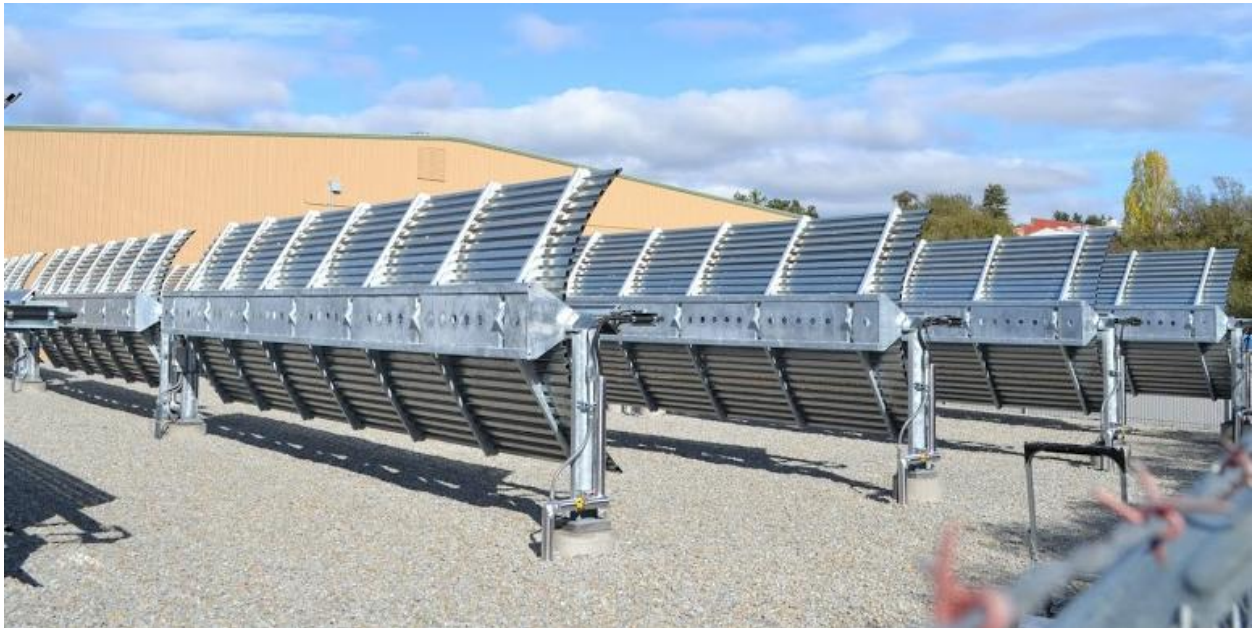
Figure 30: Sonoma Wine Company's Cogenra Solar Panels, Source: http://guntherportfolio.com/2010/11/in-search-of-cogenra-solar/
